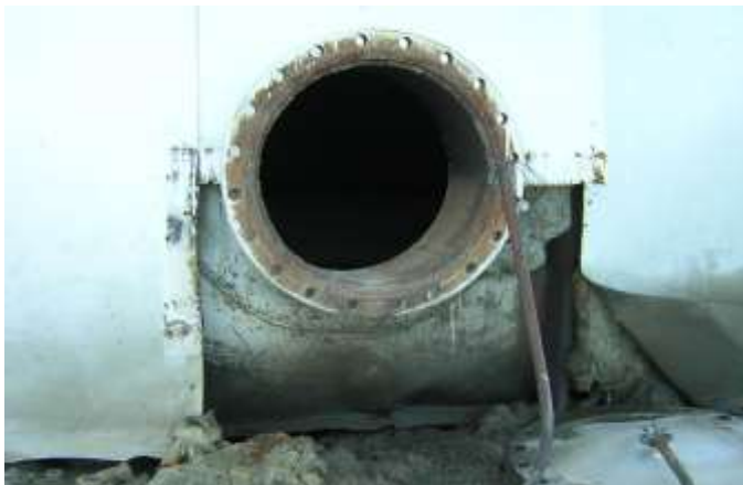
Figure 3. Wall deformation RVS-700.
