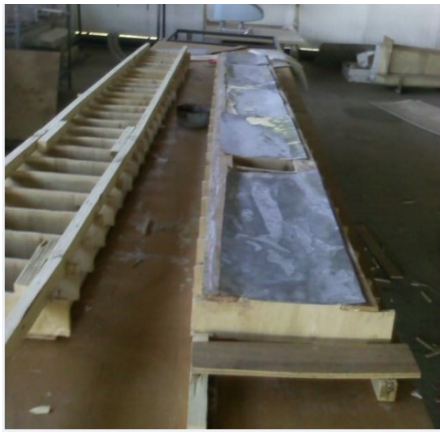
Step 10 Reinforcing the sheet at the bottom side using sufficient number of chopped strands matt layers
