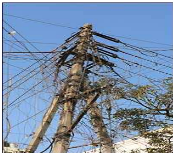
Fig:2 Illegally Tapping into the Power Line
