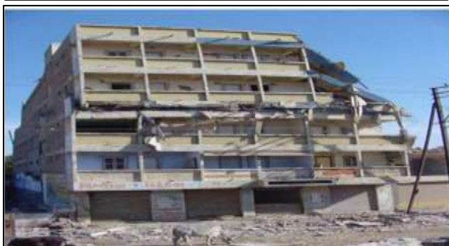
Fig 3. Earthquake effected building due to soft-storey
