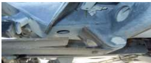
Figure 1.1. Broken spring in the front axle.
