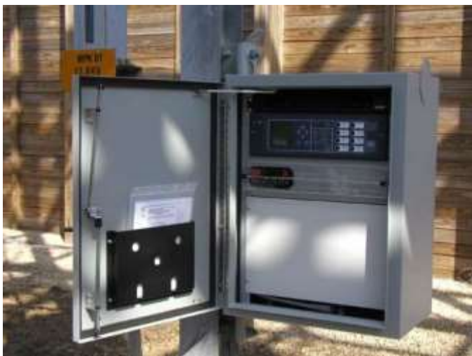
Fig. 7. A smart, automated, and distributed device installed local to the grid apparatus that it protects, controls, and manages
